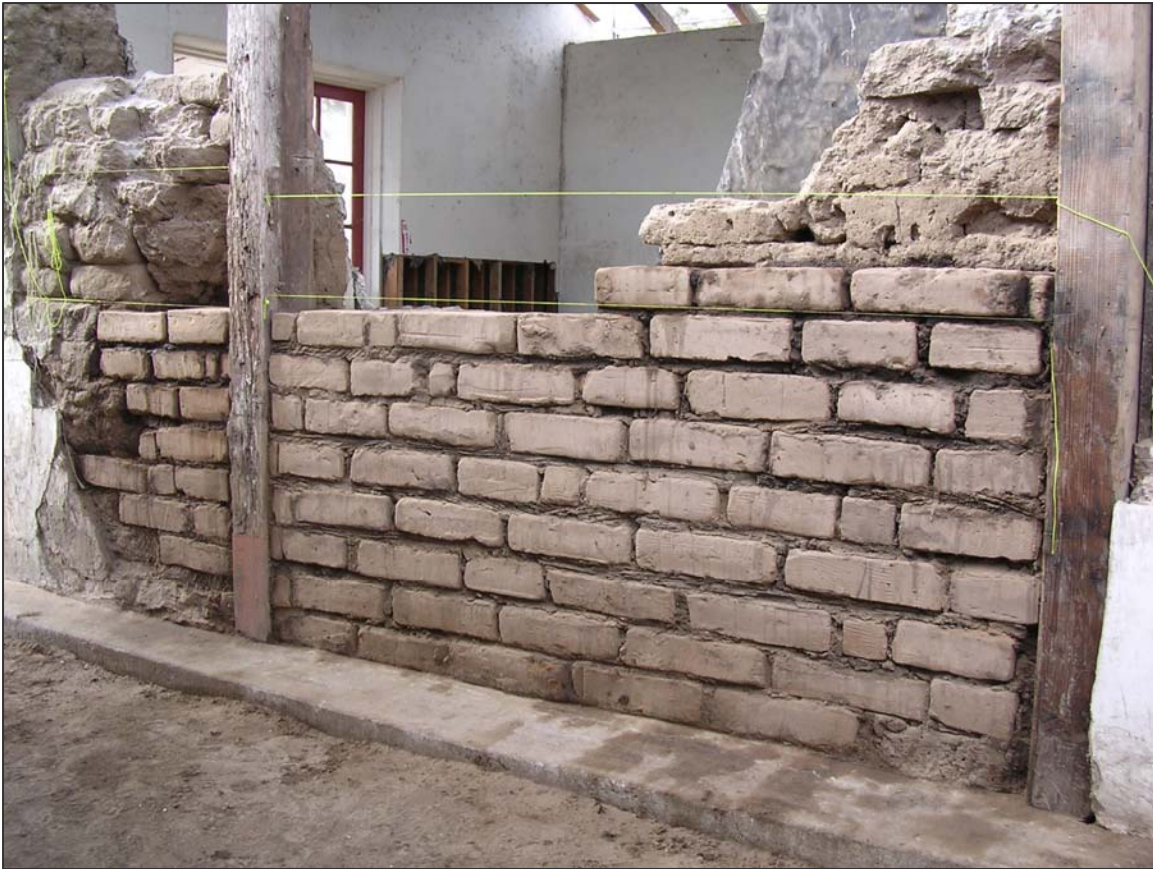
After removing concrete infills, the crew made repairs using adobe bricks. New adobes were carefully “laced” into existing work for maximum wall stability.
