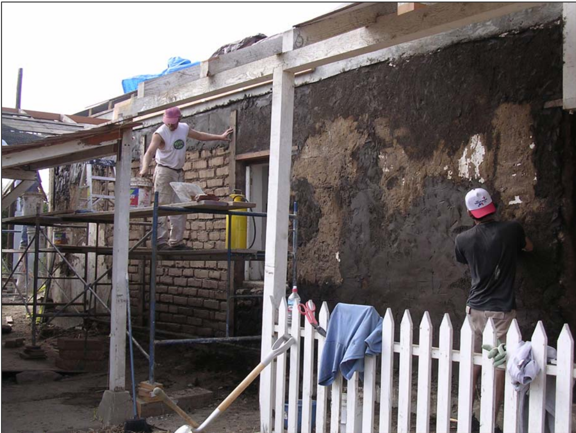
Following adobe repairs, traditional plasters and finishes were reinstated. Here, crew members are applying an earthen plaster; large areas of conserved plaster and limewash finish are visible to the right of the scaffolding.
